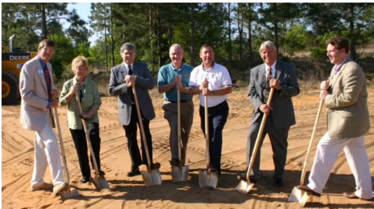
Dignitaries turning golden shovels of soil at the South Clermont Connector groundbreaking ceremony included (left to right) Jim Stivender, Jr., Director of the Lake County Department of Public Works, Lake County Commission Chairman Catherine C. Hanson, City of Clermont Mayor Pro Tem Keith Mullins, City of Clermont Council Member Ray Goodgame, Lake County Commissioner Bob Pool, City of Clermont Mayor Harold Turville, Jr. and T.J. Fish, Executive Director of the Lake~Sumter Metropolitan Planning Organization.
